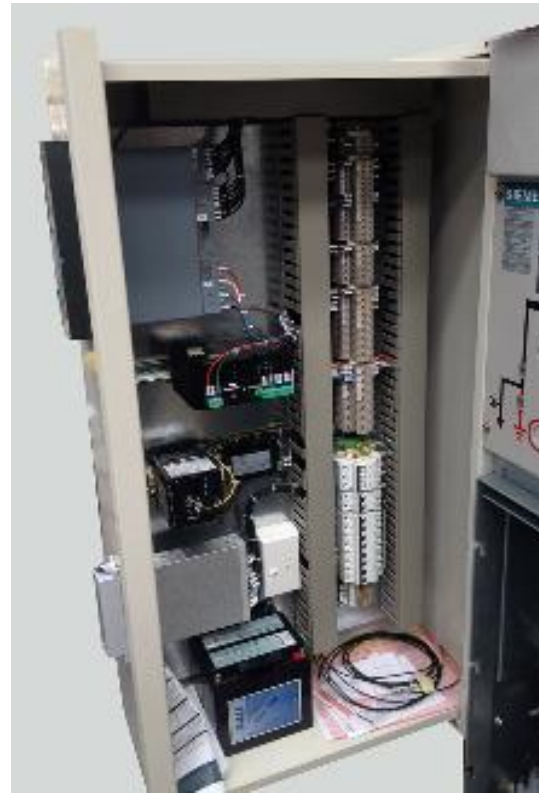
Figure 11. Automation cubicle opened.
